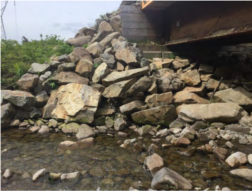
Eroding riprap downstream right abutment
