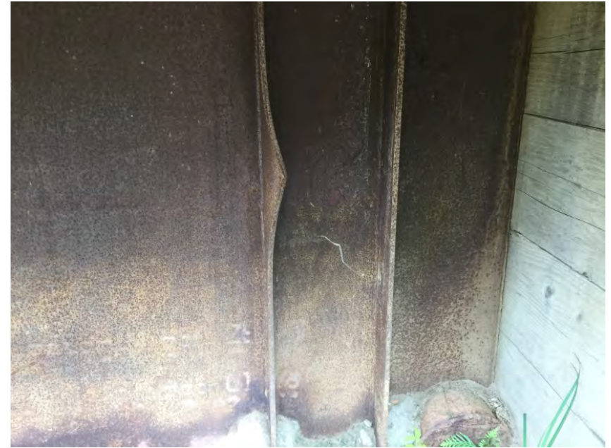
Damage noted to stiffener on downstream left abutment girder
